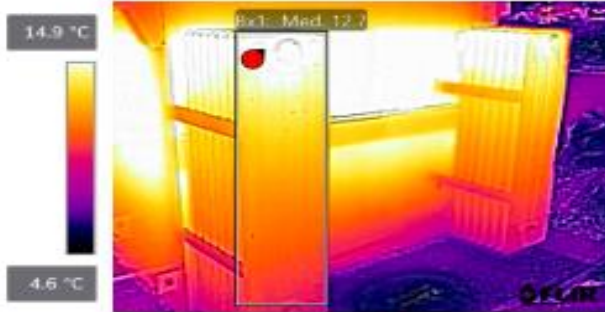
Main transformer pic4 - thermal.jpg
