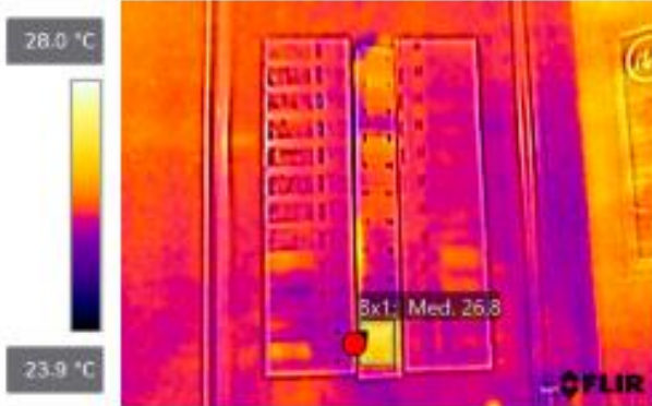
Breaker panel right of G1 - thermal.jpg
