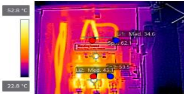
Dryer 2 disconnect pic1 - thermal.jpg
