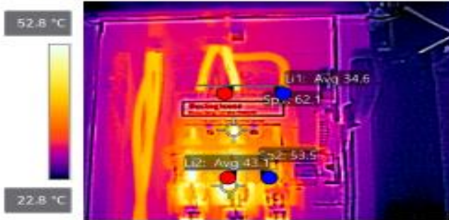
Dryer 2 disconnect pic1 - thermal.jpg
