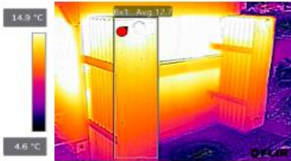
Main transformer pic4 - thermal.jpg
