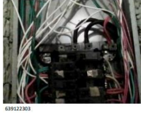
Panel #2 incoming connections and top breakers
